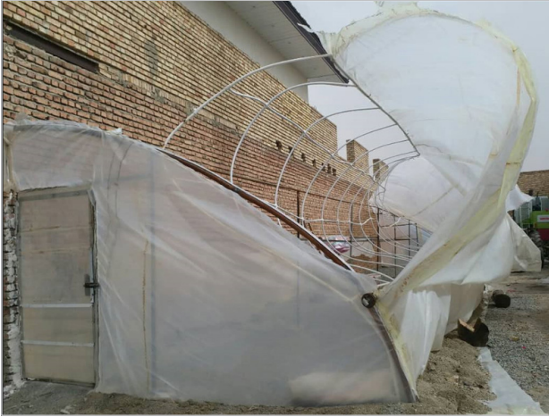
The structure and its plastic cover is dancing in the typhoon
